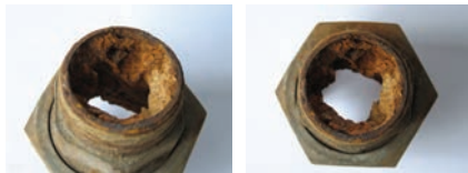
Biofilm formation on the inside of a plumbing connection
